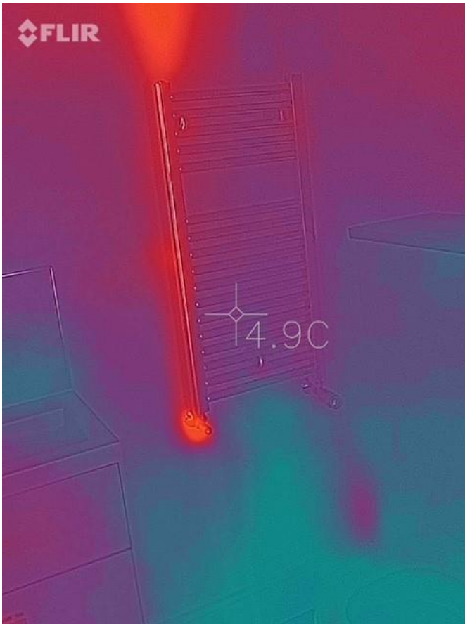
Towel radiator not heating in ensuite
